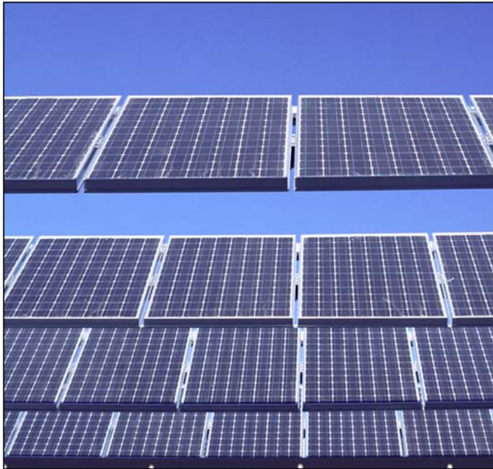
Solar Power (Photovoltaics)
