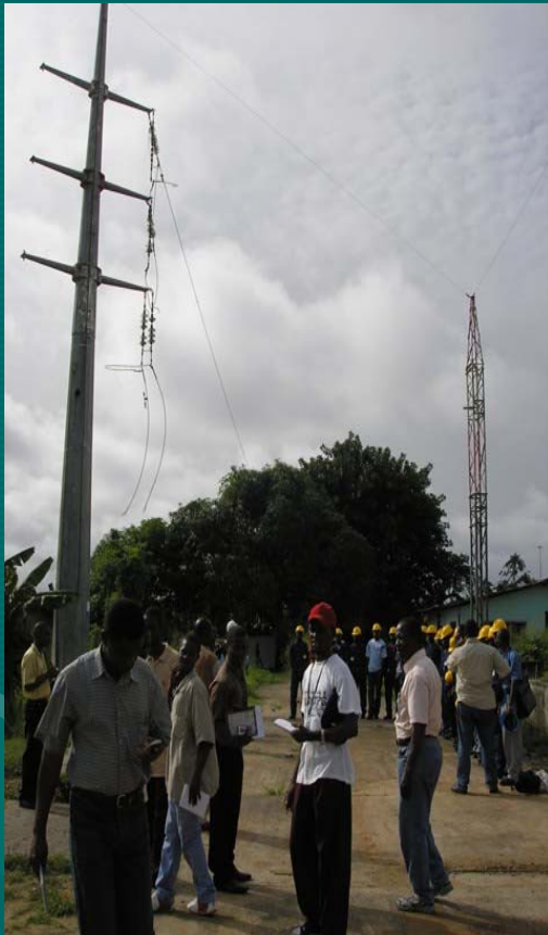
Damaged poles & lines
