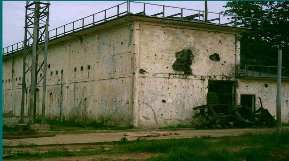
Damaged power substation
